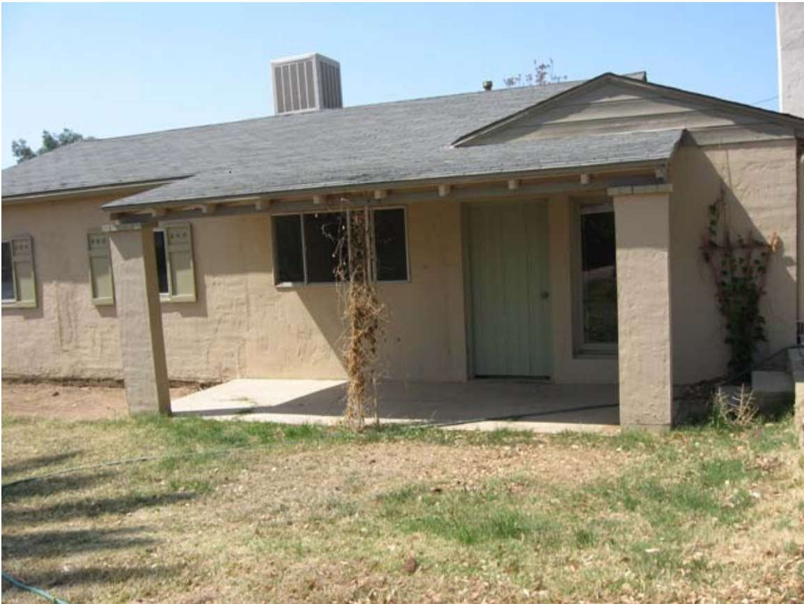
Front: FauxMasters is resurfacing the stucco with amber-gold washes same as Sylvester Stallone's mansion; A structure to cover the air conditioning system was designed by architect to mimic the old well house on the property. We plan to take out the cracked concrete and replace with a new concrete porch the full length of the front and the West side. Free-standing shade cover to extend from covered porch and wrap around house over concrete porch.
